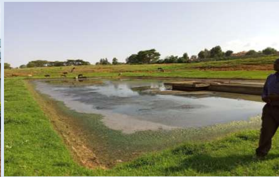
Sedimentation pond at Bungoma WWTP
